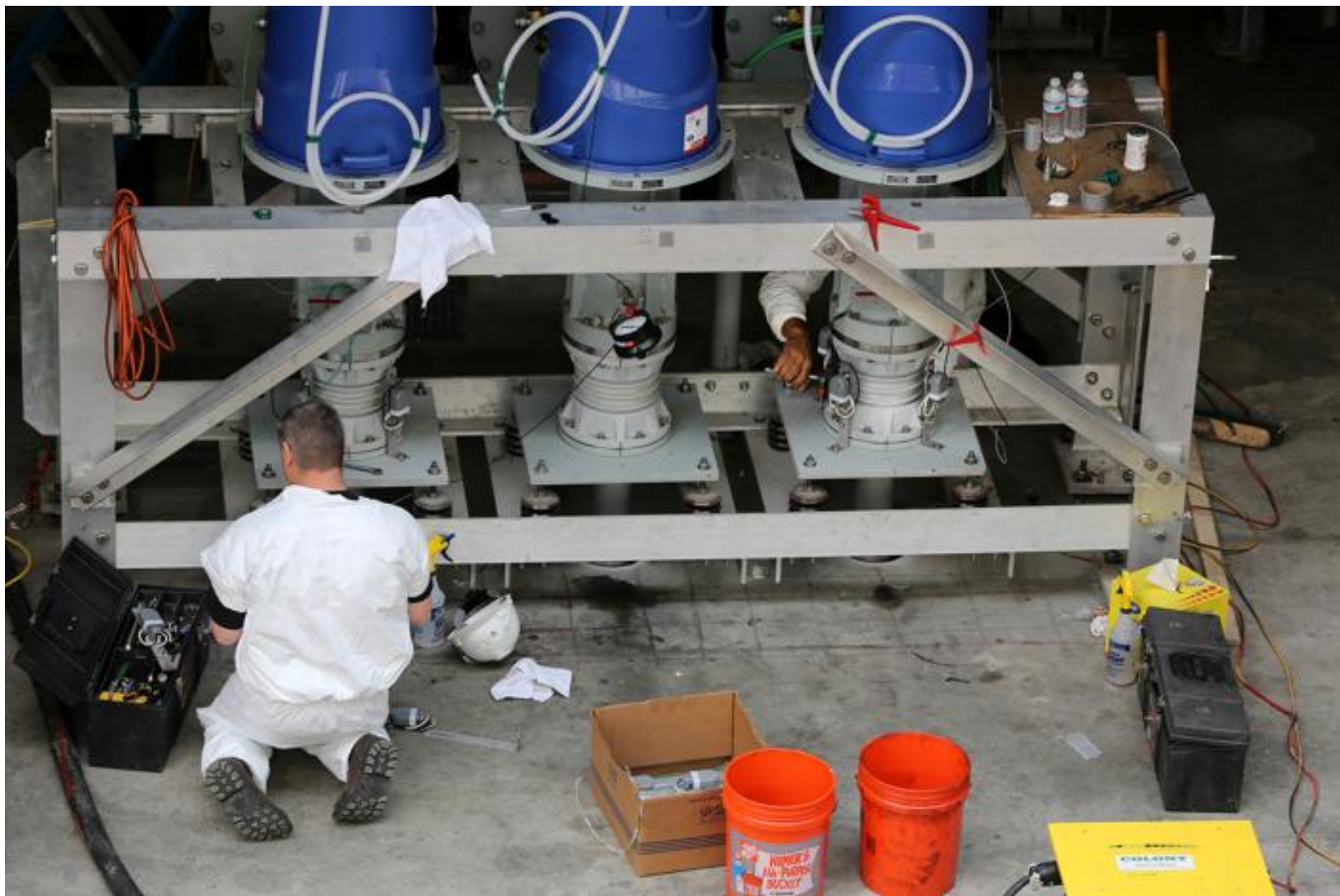
Work was done at a power station in the Back Bay last summer after an outage affected the Boston neighborhood. Credit: (Pat Greenhouse/Globe Staff)
