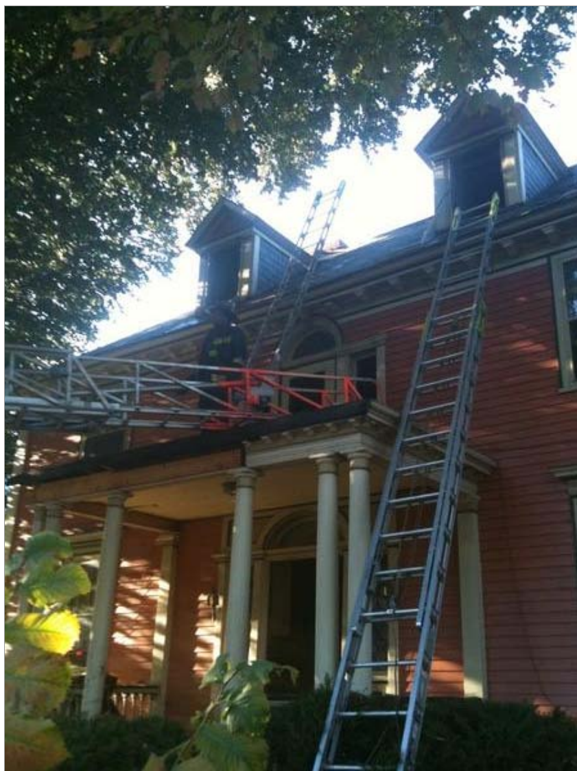
(Courtesy Boston Fire Department)
