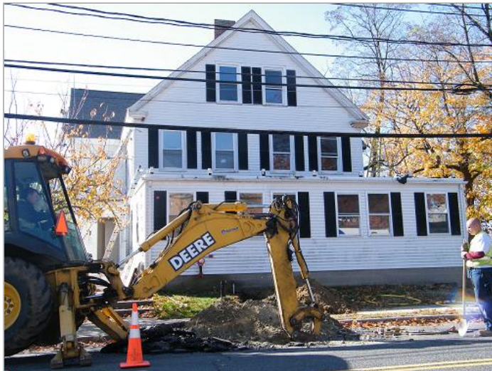
A new gas line for the Larry's Place building on Lincoln Street was being installed Wednesday as one of the final steps before an open house next week. Residents are expected to move in by early December. (Matt Rocheleau for The Boston Globe).
