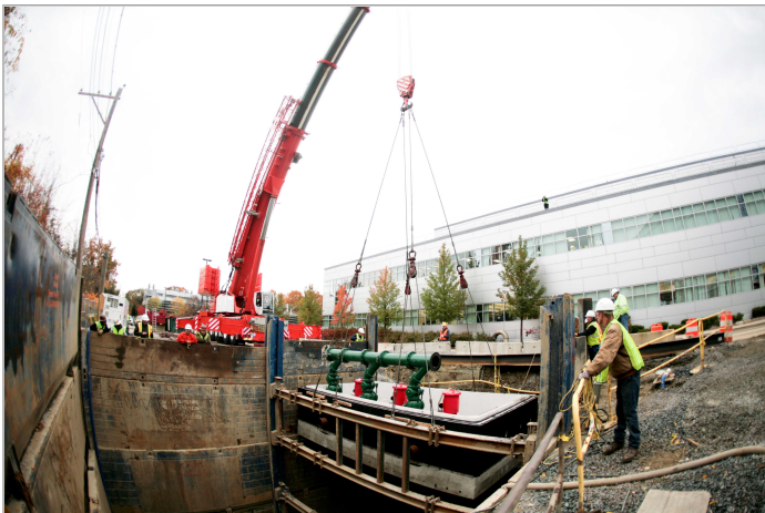
Work crews lower the first piece of the new Framingham wastewater pumping station into the ground on Oct. 27. (Courtesy: Massachusetts Life Sciences Center)
