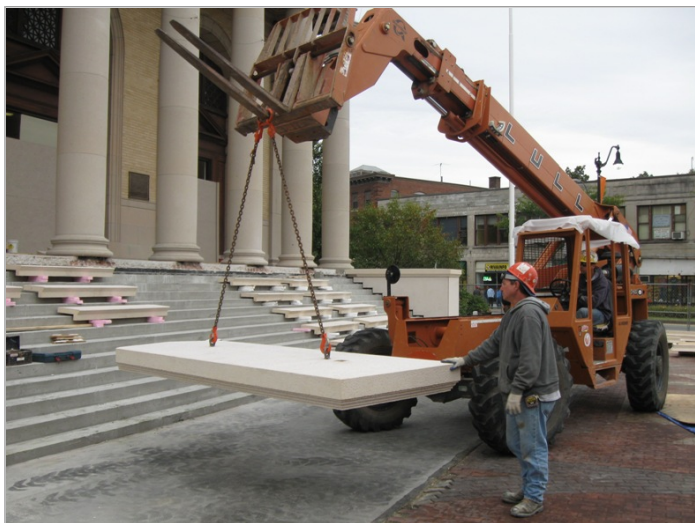
Recent construction on the stairs of Memorial Building's main entrance. (Courtesy: Town of Framingham)
